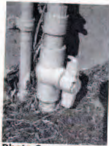
Photo 8 Main water shut off
