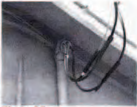
Photo 35 No drip loop
