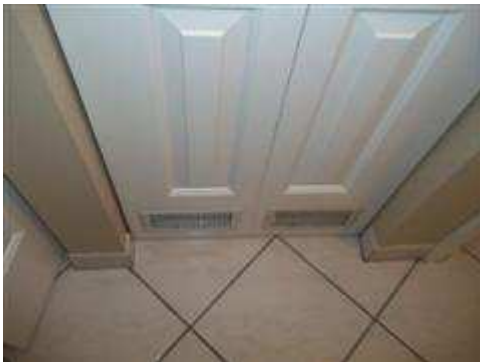
An auxiliary intake was installed in the laundry room and the wall voids were not sealed allowing air from that area to be drawn into the system.
