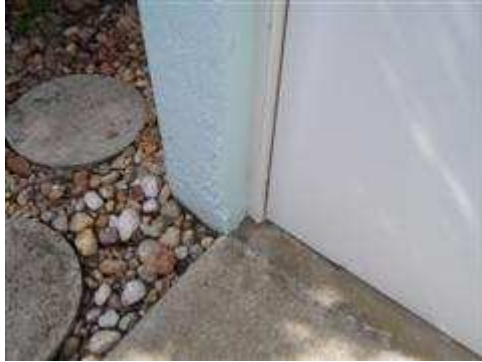
Rear garage door and frame were rotted (replace).
