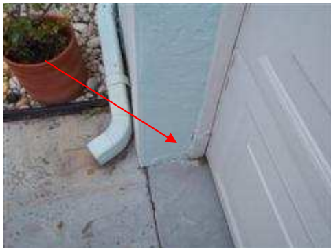
Main garage door trim was damaged at both sides.
