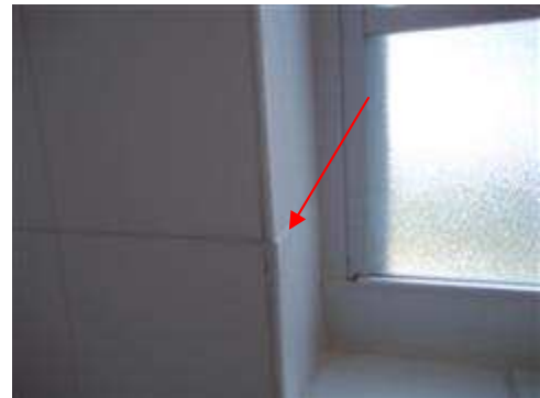
Tiles in hall bathroom shower around window were missing grout.
