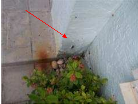
Damaged stucco observed at front entrance.
