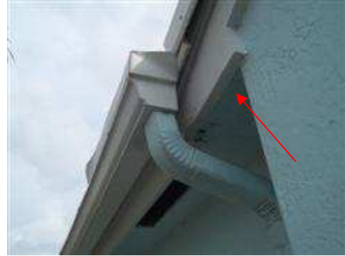
There were numerous areas of rotted fascia observed around the home.
