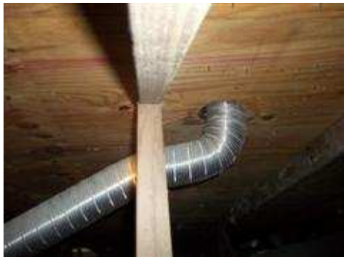
Lint removal line was ribbed conduit and smooth conduit is required. The ribbed lines may allow lint to collect in areas and block the airflow which may lead to poor dryer performance and possibly a fire.
