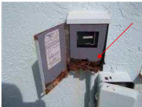
Service disconnect box for pool equipment was rusted out.
