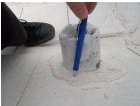
The vent stack at the front of the home was too low (six inches is the minimum height)
