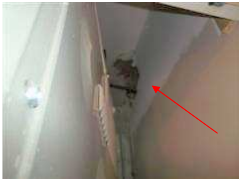
Damaged wall exposing plumbing connections at kitchen viewed when the stove was moved.
