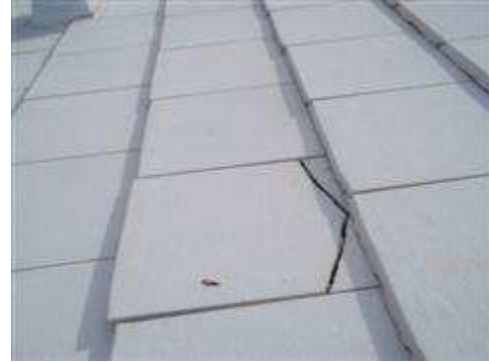
Broken roof tile observed on main roof.
