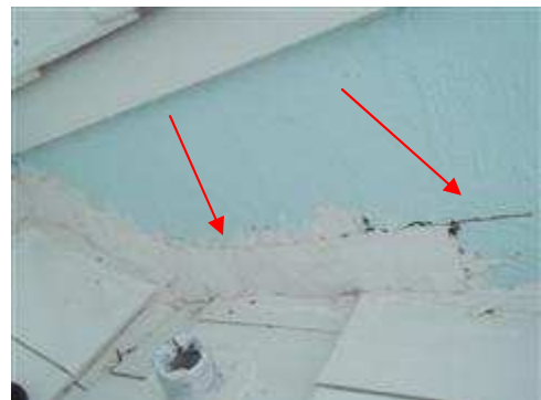
During the flashing replacement over the front entrance, the wall was not repaired properly.
