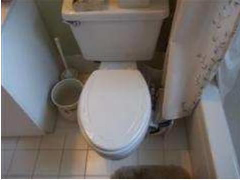
Toilet was loose at floor with probable damaged wax ring in hall bathroom.
