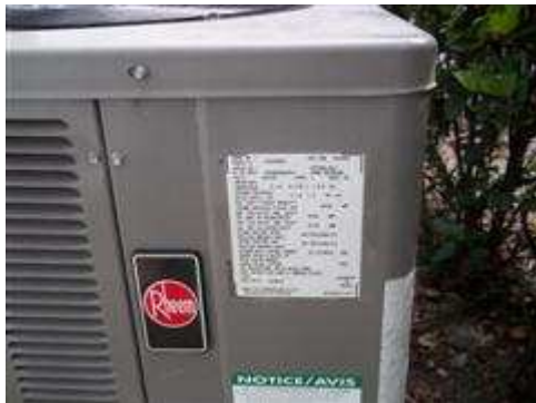
Condensing unit data plate.
