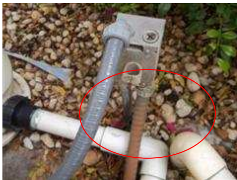
Support post for pool equipment was rusted out .
