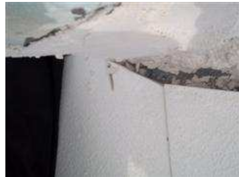
Upper level gutter downspout was not present and water has washed away the cement on the lower portion of the roof. Over time, this will most likely turn into a roof leak.
