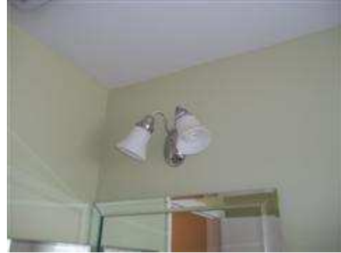
Light in hall bathroom shut off when the G. F. I. receptacle was tripped.
