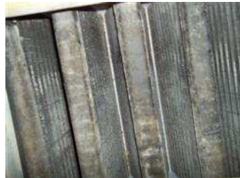
Coils were dirty/clogged at air handler restricting air flow.
