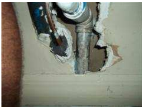
Damaged wall observed in air handler closet.
