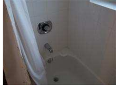
Water was coming out of the shower and tub spout in the hall bathroom at the same time.
