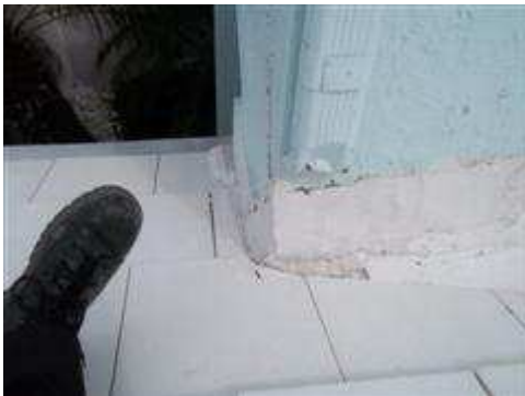
Upper level gutter downspout was not present and water has washed away the cement on the lower portion of the roof. Over time, this will most likely turn into a roof leak.
