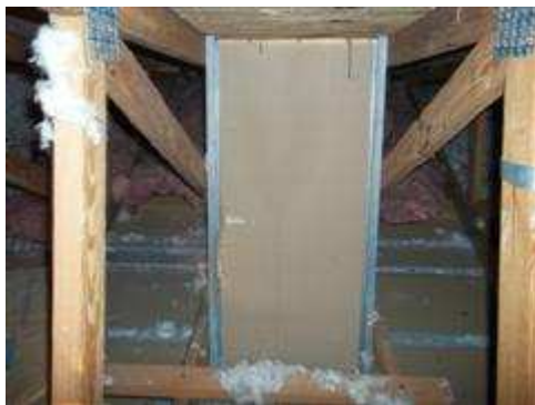
Insulation was not present at skylight and surrounding areas of attic.
