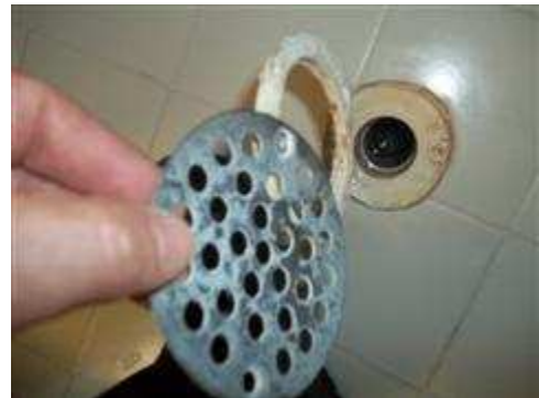
Shower drain assembly was not attached in the master bathroom.
