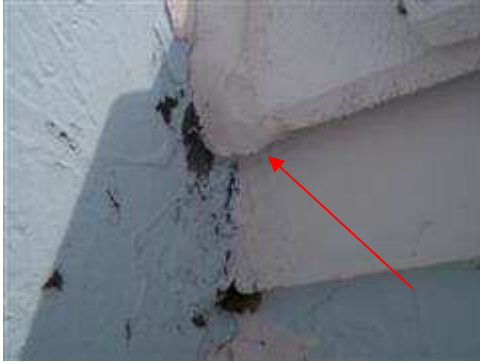
Damaged fascia observed at front entrance on second level of the roof.
