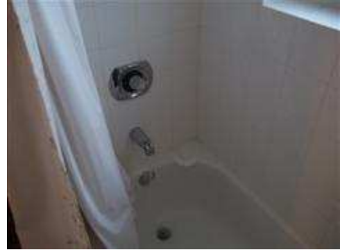
Water was coming out of the shower and tub spout in the hall bathroom at the same time.
