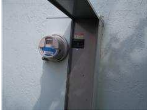
Main service disconnect at right side of house.
