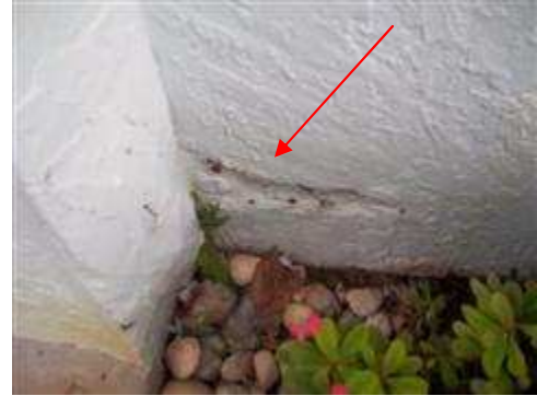
Damaged stucco observed at front entrance.
