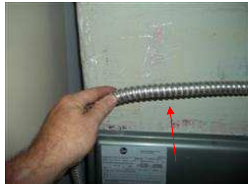
Conduit for air handler was not secured.
