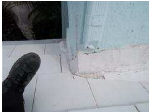
Upper level gutter downspout was not present and water has washed away the cement on the lower portion of the roof. Over time, this will most likely turn into a roof leak.
