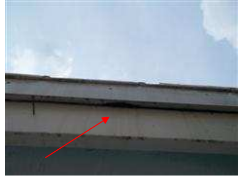
Damaged drip edge observed at left side of house.
