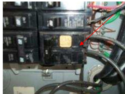
There was another manufacturers breaker present in the Challenger panel. Most manufacturers do not allow this.
