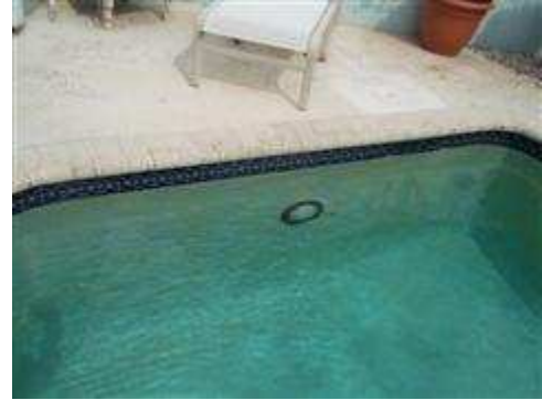
Pool light ring was rusted.
