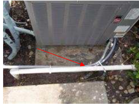
Electrical wiring for a/c condensing unit was not secured properly.
