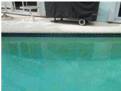
There were numerous areas of the pool coating which were deteriorating exposing the pool shell and in some instances, the pool wire/rebar.
