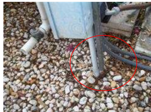
Support post for pool equipment was rusted out and conduit was damaged.
