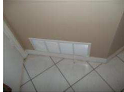
An auxiliary intake was installed in the laundry room and the wall voids were not sealed allowing air from that area to be drawn into the system.
