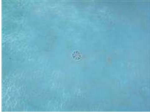
Improper drain grate observed in pool.
