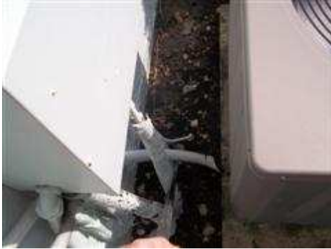
Heat recovery system has been disconnected from the air conditioner. (removal is recommended).
