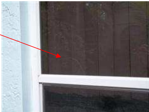
Right side window had cracked glass.
