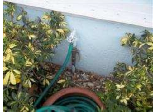
Main water shut off at front of house.
