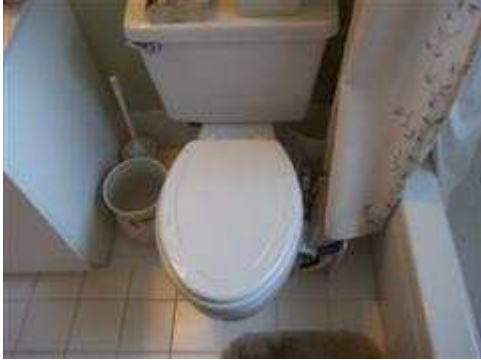
Toilet was loose at floor with probable damaged wax ring in hall bathroom.
