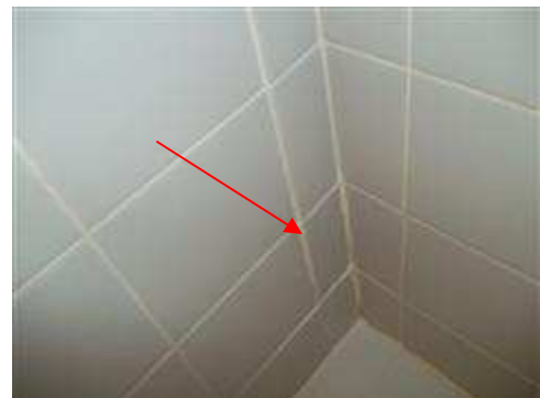
Tiles were loose at interior and exterior master bathroom shower walls with missing grout.
