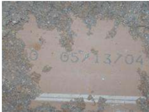
Water meter in basement.
