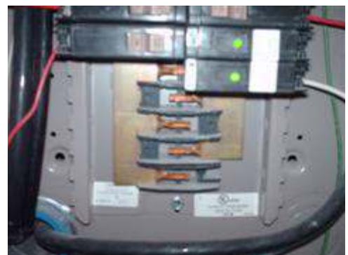
Electrical panel in basement.
