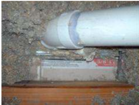
Grounding pipe for water meter in basement. At ground level.
