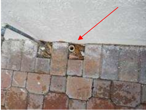
Uncapped drain line observed at rear patio.
