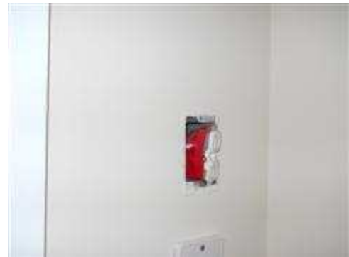
Receptacle in master bedroom was not secured to box.
