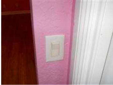
Switch was broken in left rear bedroom.
