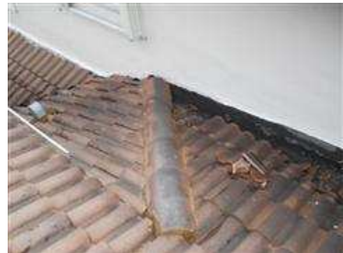
Deteriorated roof covering observed at transition between the second story and the first story roof.
