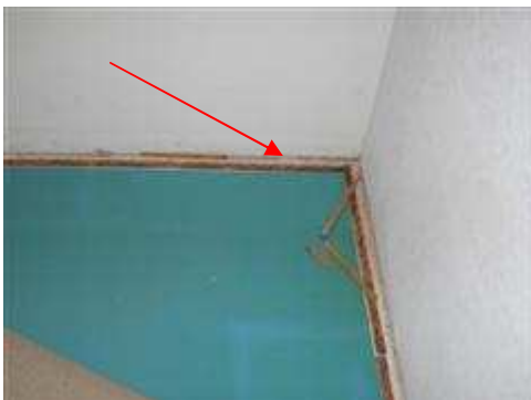
Staining observed at master bedroom closet behind air handler.
