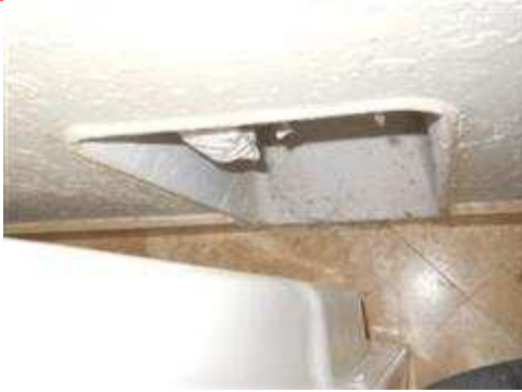
Dryer lint line was not attached to dryer.
