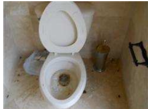
Toilet in Cabana bathroom did not shut off.
