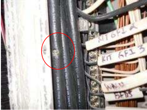
Damaged insulation observed to the panel box feed lines in both panels behind the dead front cover retaining screws.
