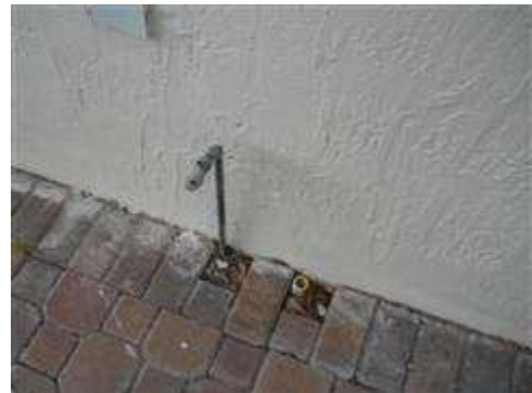
Plumbing line at rear of home was not secured.
