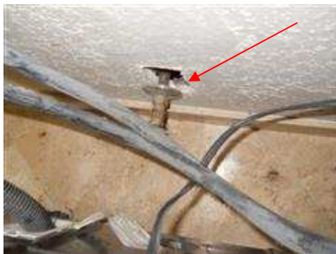
Water line was not secured in back of washing machine. This line may not be permitted to be in this location.
