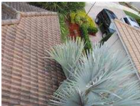
Tree at the left side of the home was up against the house and interfering with the roof.
