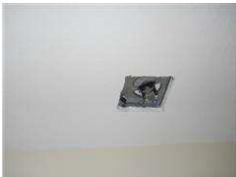
Cover for vent fan in addition bathroom was not present. This fan also does not appear to exit to the exterior as required.
