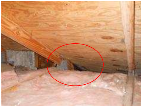
Roof leak observed at garage with damaged decking.
