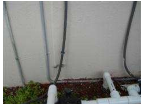
Conduit for pool equipment was not secured properly.
