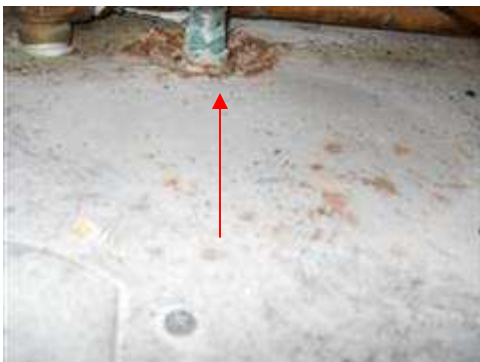
The water heater was rusted out at the inlet lines.
