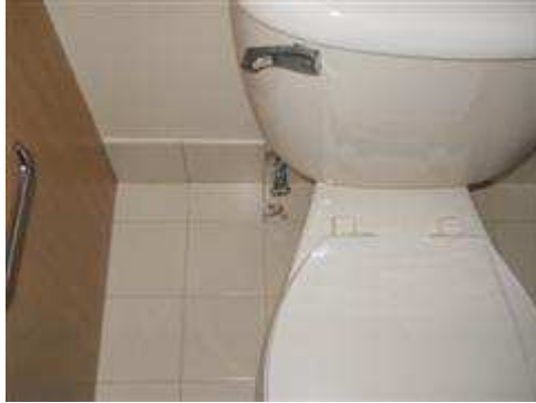
Shut off valve for upstairs toilet was leaking. Toilet was loose at floor with a possible damaged wax ring.
