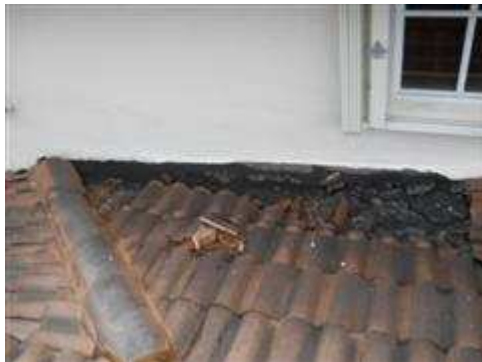
Deteriorated roof covering observed at transition between the second story and the first story roof.
