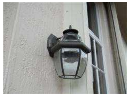
Rear patio light fixture was not secured/sealed properly.
