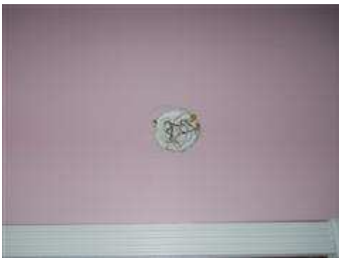
Light fixture was not present in left rear bathroom exposing wiring.
