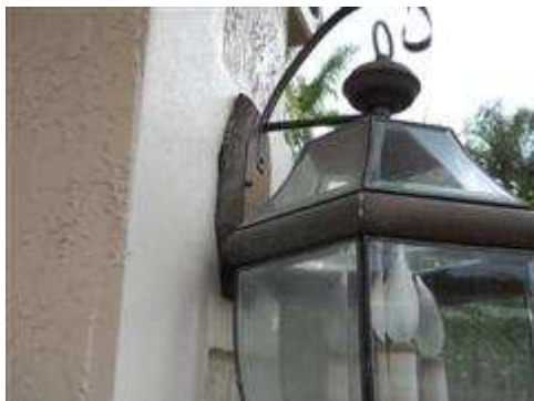
Front light fixtures were not secured/sealed properly.
