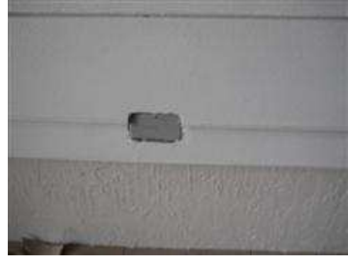
Receptacle at front entrance was recessed in the decorative banding and access was limited.
