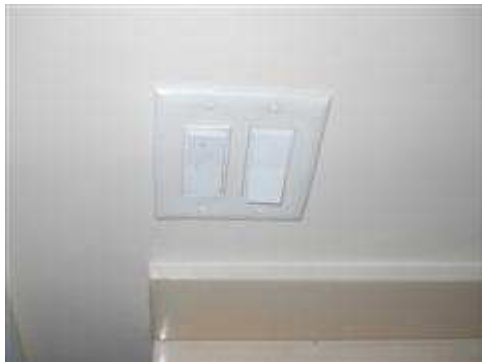
Switch was broken in upstairs bathroom.
