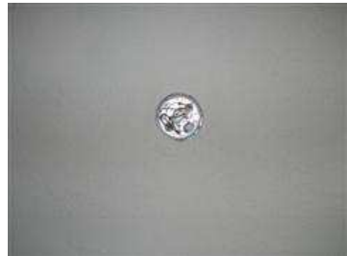
Missing light fixtures in den exposing wiring.
