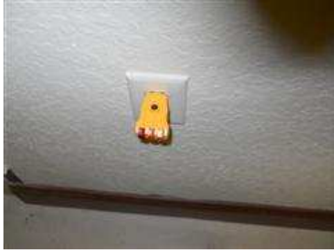
Receptacles in garage were not G.F.I. protected.
