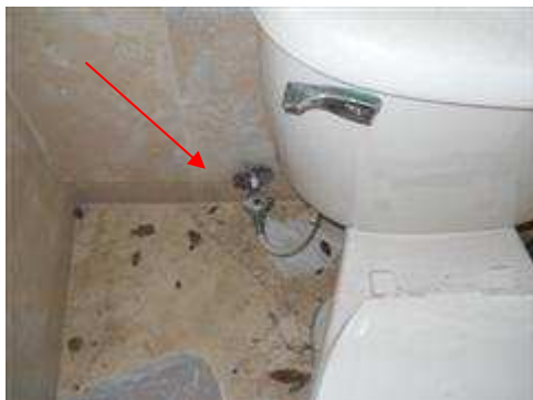
Shut off valve for toilet in Cabana bathroom was leaking.
