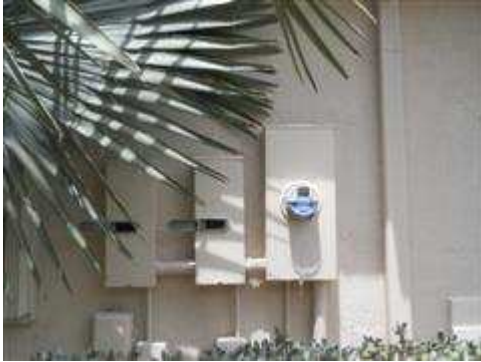
Main service disconnects at left side of house.
