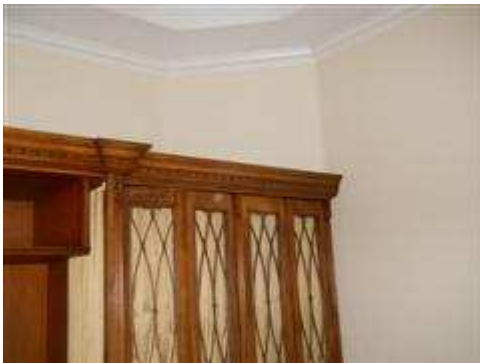
Master bedroom window was dry-walled over.
