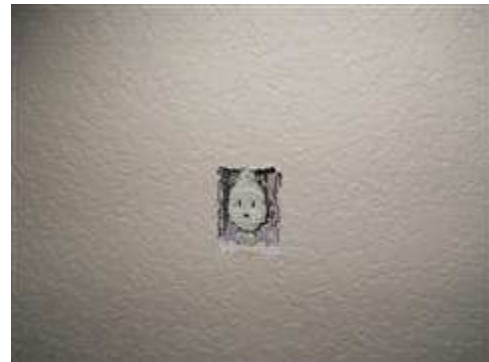
Face plate was not present at receptacle in garage hall exposing wiring.
