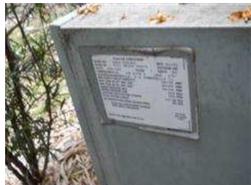
Condensing unit data plate.
