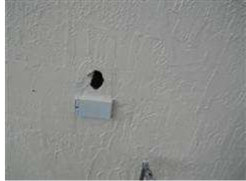
Damaged wall observed at rear patio.
