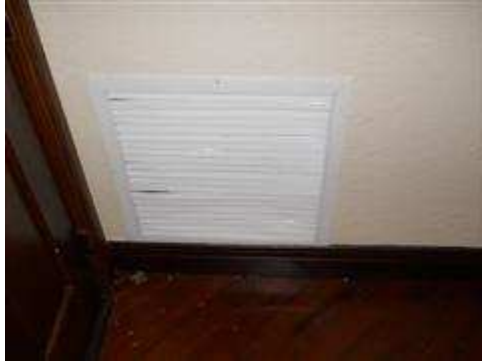
Intake grill in the master bedroom was installed in a manner that when the door is open, the flow to the unit is blocked.
