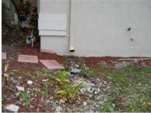
Improperly terminated gutter downspout at right side of house has washed away a large amount of soil.
