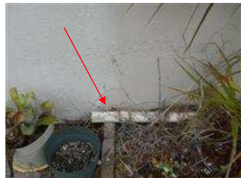
Uncapped drain line observed at rear patio.
