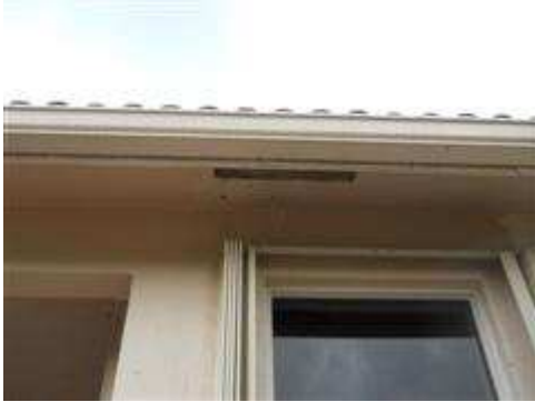
Exposed wiring at rear of house.
