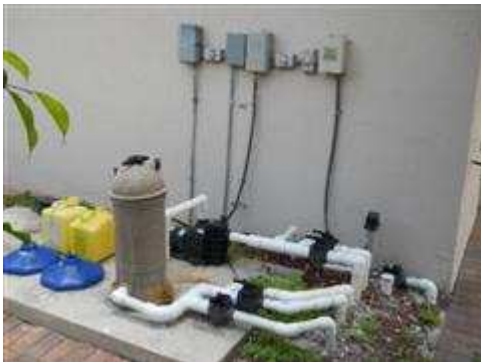
Pool equipment (not tested).
