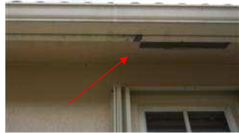
Damaged fascia observed at right side of house.
