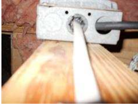
Improper junction observed at attic light switch box.
