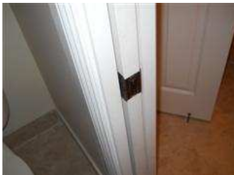
Pocket door did not lock at left side middle bathroom.
