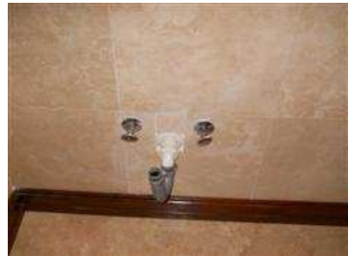
Sink was not present in left side half bathroom.
