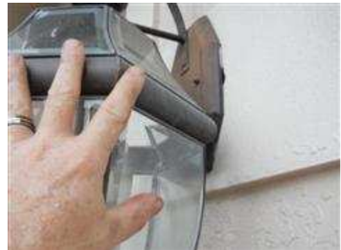
Front light fixtures were not secured/sealed properly.
