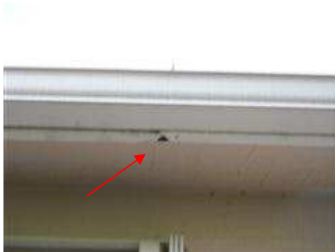
Damaged fascia observed at left side of house.
