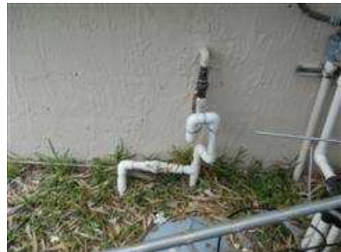
Main water shut off at left side of house.
