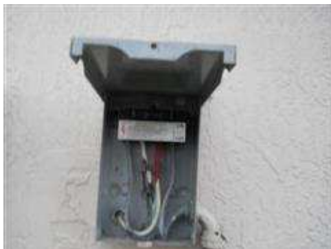
Inner cover plate was not present at two a/c condensing unit disconnects exposing the lugs and wiring.
