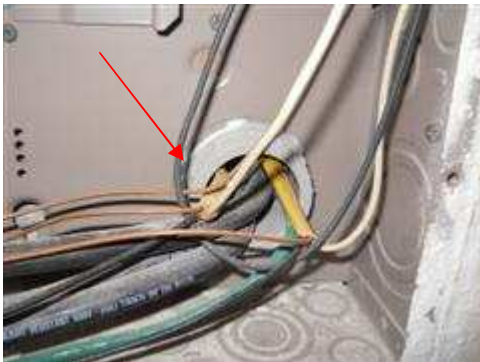
Wiring for what is labeled landscape lighting, was routed through the main feed conduit.
