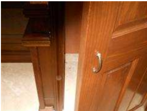
There was no latching mechanism present for the front den closet door.
