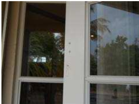
Pool alarm sensors were not present at rear patio doors. Other sensors require batteries.
