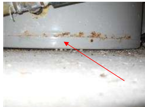
The base of the water heater was rusted out.
