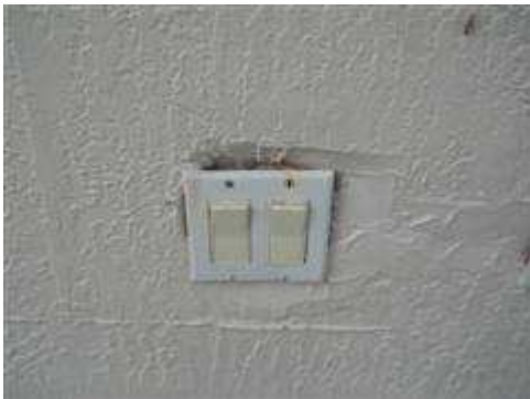
Damaged wall observed at rear patio.
