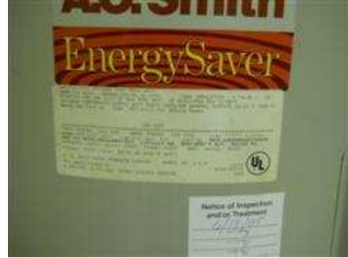
Water heater data plate.
