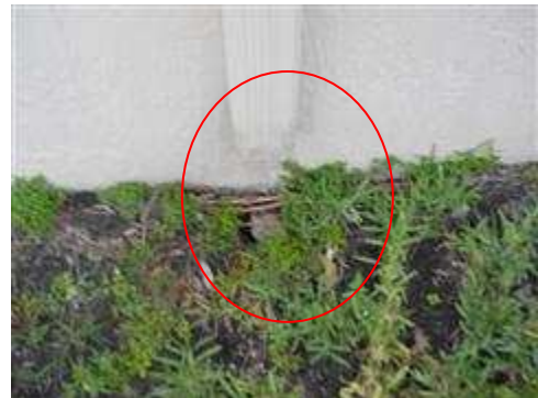
Missing gutter downspout which has caused the soil to erode at the left side of the house.
