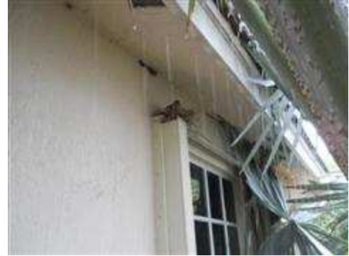
Tree at the left side of the home was up against the house and interfering with the roof.
