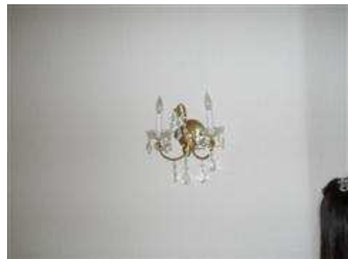
Lights in dining room did not function.
