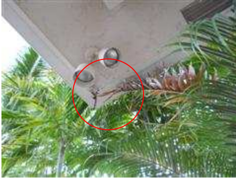
Damaged fascia observed at right rear corner of house.
