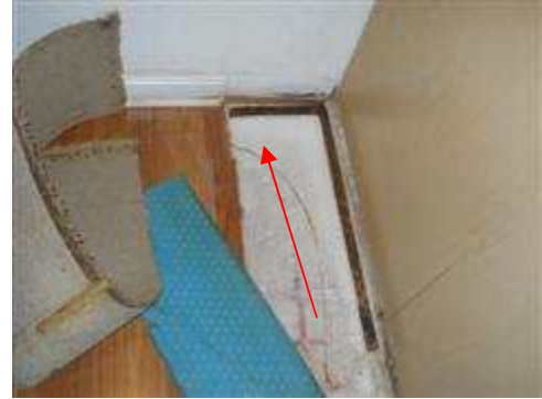
Damaged wall/baseboard observed in left side closet.
