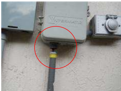
Conduit at pool pump timer was not attached to box properly.
