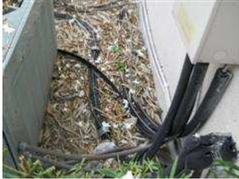
Insulation was damaged at the refrigerant lines for the a/c condensing units.
