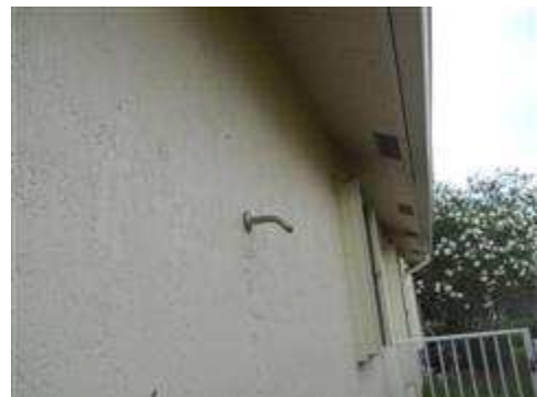
Shower head was not present at rear patio shower.
