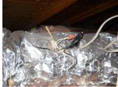
Open junction observed at garage attic for inline fan for the addition bedroom duct work, which did not shut off.
