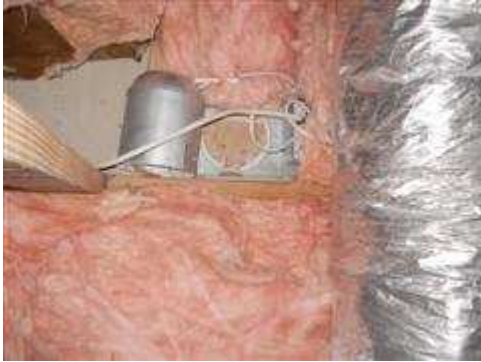
There were several high-hat lights that appeared to be functional laying on the attic floor.
