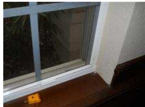
Window in den did not stay open (springs).
