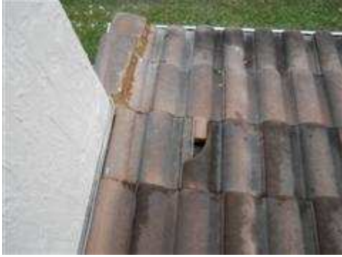
Broken tiles observed on main roof.
