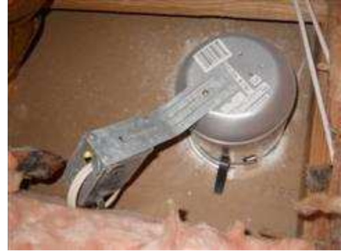
Improper connection observed at master bedroom high-hat light.
