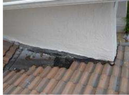
Deteriorated roof covering observed at transition between the second story and the first story roof.
