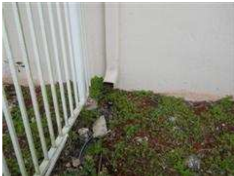
Improperly terminated gutter downspout at right side of house has washed away a large amount of soil.
