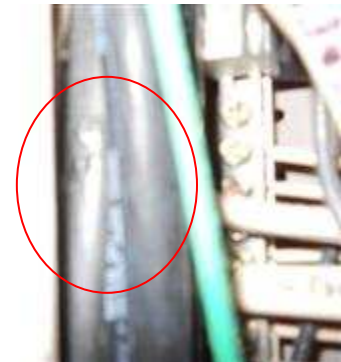
Damaged insulation observed to the panel box feed lines in both panels behind the dead front cover retaining screws.
