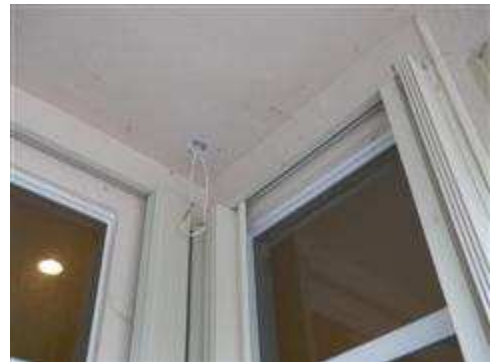
Exposed wiring observed at rear patio.
