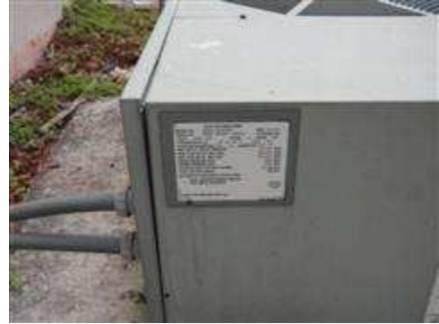
Condensing unit data plate.
