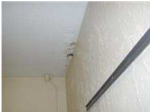
Damaged ceiling observed in garage from active roof leak.
