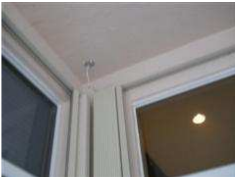
Exposed wiring observed at rear patio.
