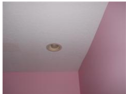
Lights did not function in left rear bathroom.
