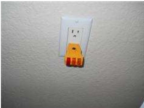
Receptacle in the hallway leading to the garage showed reverse polarity.
