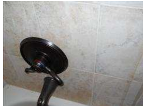
Shower handle in left side middle bathroom had no stopping point.
