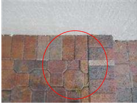
The landing area at the rear patio shower had several pavers which sunk when stepped on.
