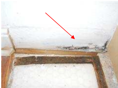
Damaged wall/baseboard observed in left side closet. Fungus was present as well.
