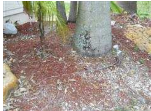
Exposed wiring observed in numerous areas of the yard for the landscape lighting.
