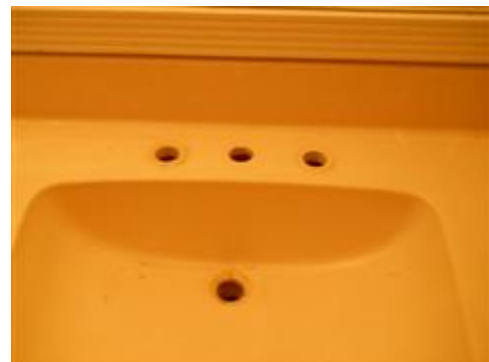
Faucets and drain lines were not present at left side middle bathroom.
