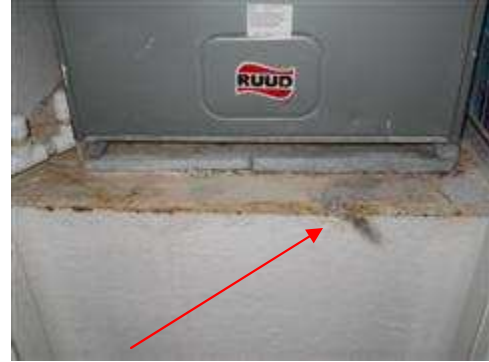
Shelf/box for left side air handler was damaged. Fungus was present as well.
