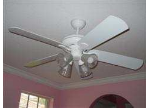
Fan did not function in left rear bedroom.
