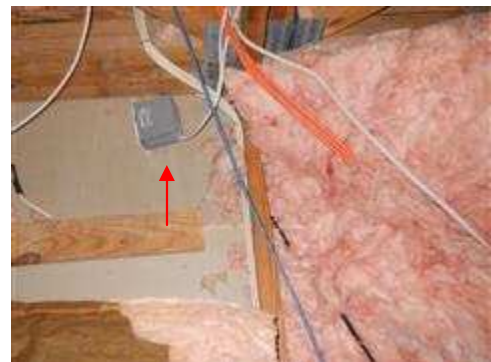
Un-mounted junction box, possibly a light switch observed in the attic.
