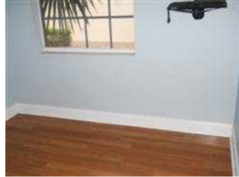
There was no receptacle present at the left side wall in the addition bedroom.
