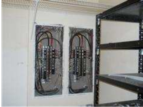
Breaker panels in garage with covers removed.
