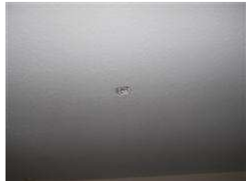
Light fixture was not present at upstairs bedroom exposing wiring.
