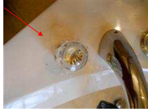
Hot water faucet was leaking at the master bathroom tub.
