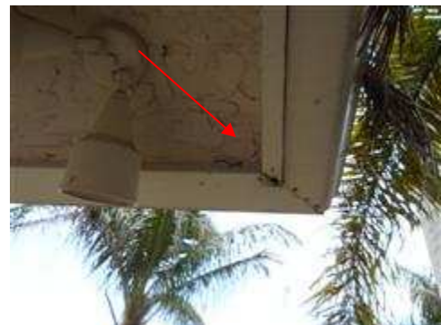
Damaged fascia observed at right front corner of house.
