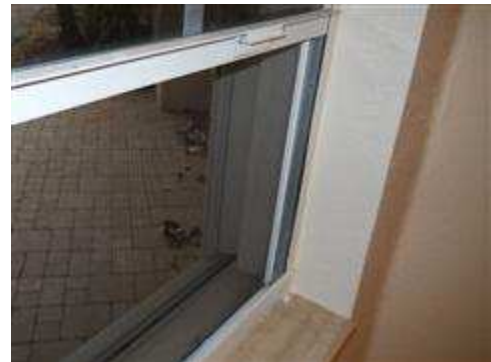
Spring was broken at dining room window.
