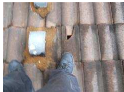
Broken tiles observed on main roof.
