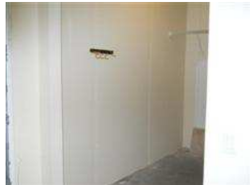
The smaller garage door was walled over and not accessible.
