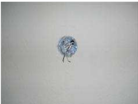
Missing light fixtures in den exposing wiring.
