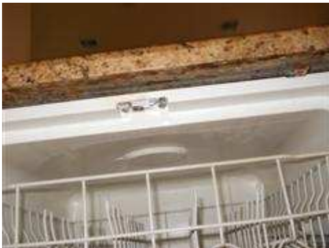
Dishwasher was not mounted and was not tested.
