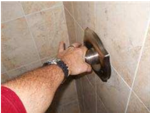
Shower fixtures were not secured in the left rear bathroom.
