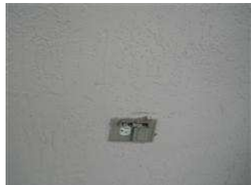
Receptacle at rear patio had a broken cover.
