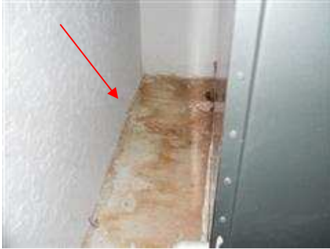
Shelf/box for left side air handler was damaged.
