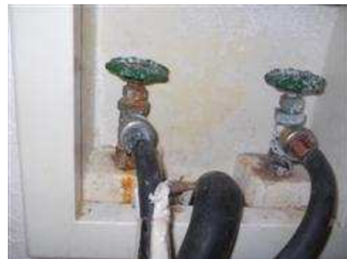
Shut off valves were leaking at washing machine.
