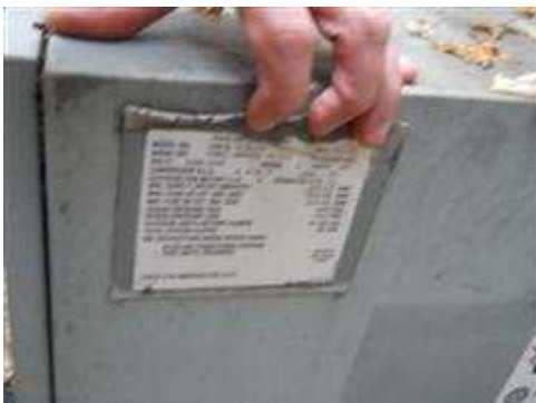
Condensing unit data plate.
