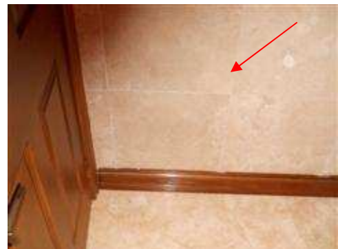
Tiles were damaged and loose at left side half bathroom wall.
