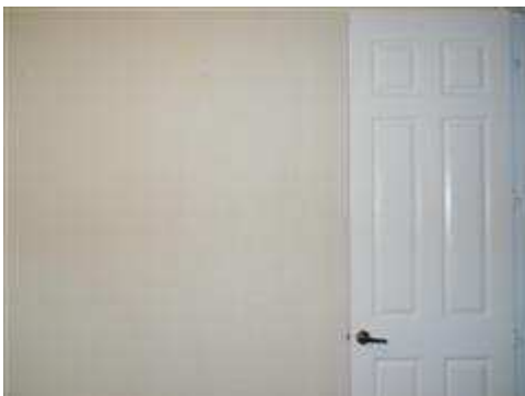
Staining/repairs observed at left bedroom wall.
