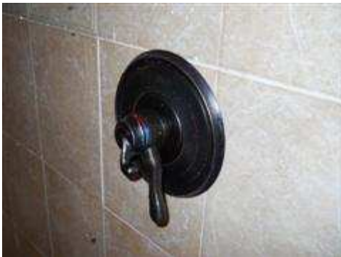
Shower handle in master bathroom was backwards (hot is required to be on the left side).
