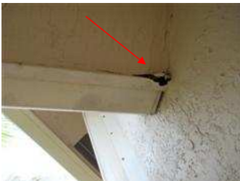
Roof leak observed at front entrance with damaged fascia.
