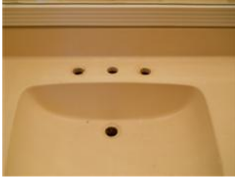
Faucets and drain lines were not present at left side middle bathroom.
