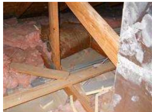
Insulation has been disturbed/improperly installed in several areas of the attics.
