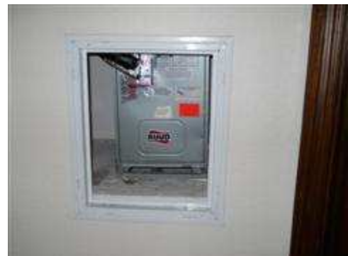
The air handler in the master bedroom was not readily accessible.
