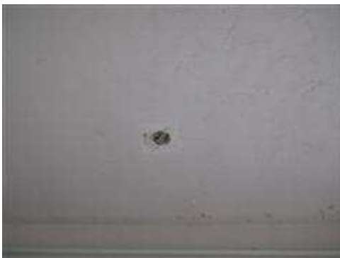
Exposed wiring observed at rear patio.
