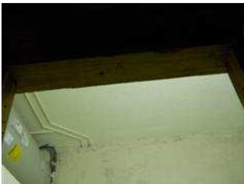
Attic access staircase in garage was installed improperly.
