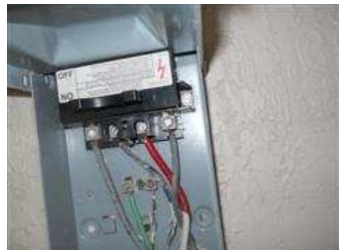
Inner cover plate was not present at two a/c condensing unit disconnects exposing the lugs and wiring.
