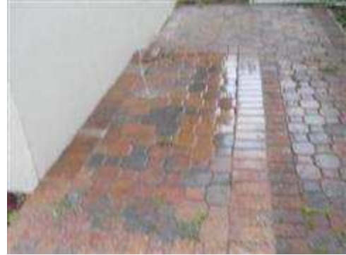
The landing area at the rear patio shower had several pavers which sunk when stepped on.
