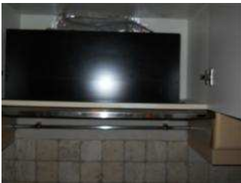
Hood fan did not function.
