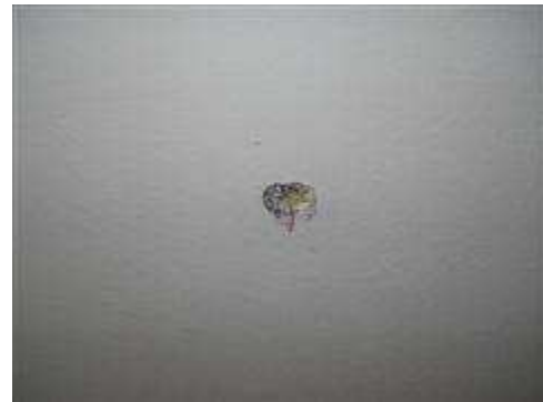
Light fixture was not present in the upstairs bedroom exposing wiring.
