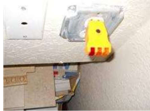
Receptacles in garage were not G.F.I. protected.
