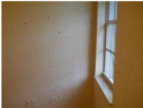
Improper repair observed at left bedroom wall behind shower.
