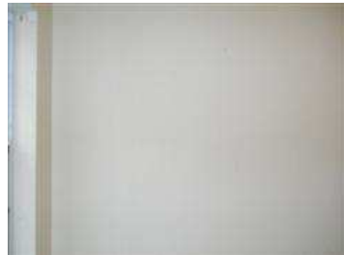
Staining/repairs observed at left bedroom wall.
