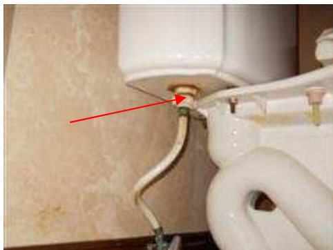
Toilet was leaking at left side half bathroom from bowl tank gasket and feed line.
