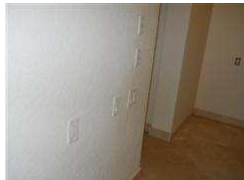
The hall between the garage and the rest of the home appears to be installed over a wood deck.
