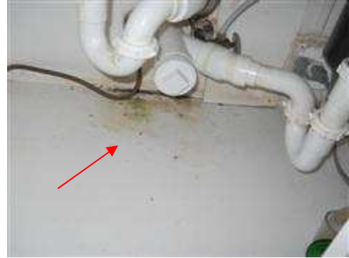
Shelf under kitchen sink was damaged.
