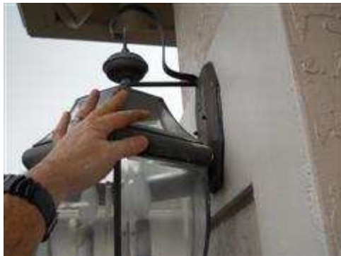
Front light fixtures were not secured/sealed properly.
