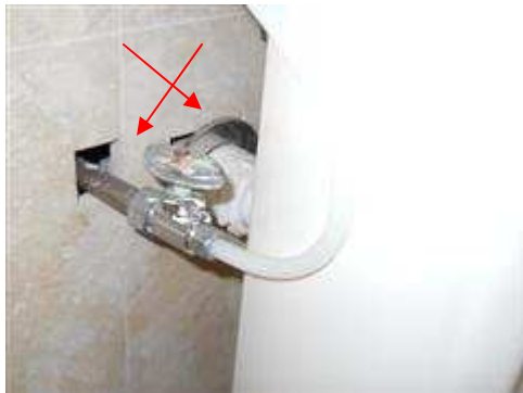
Shut off valves for "Cabana" bathroom sink were not secured.
