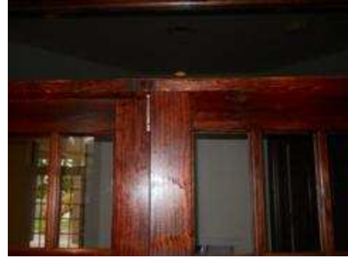
Front "den" door did not close.
