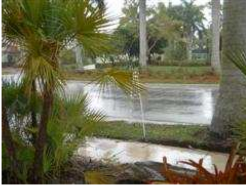
Several sprinkler heads were not present.
